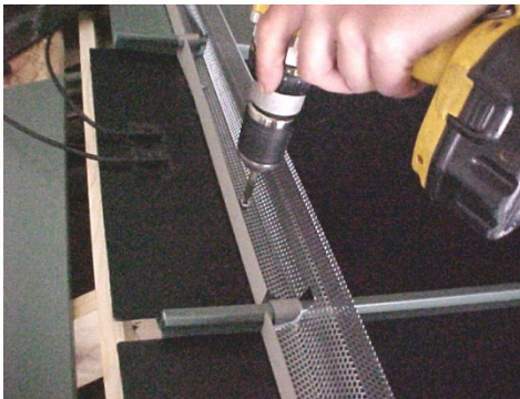
Installing Z-Closure, taking care to put screws through areas where penetrations are allowed
