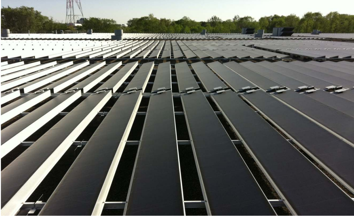
Figure 41: Installed PowerTilt Array
