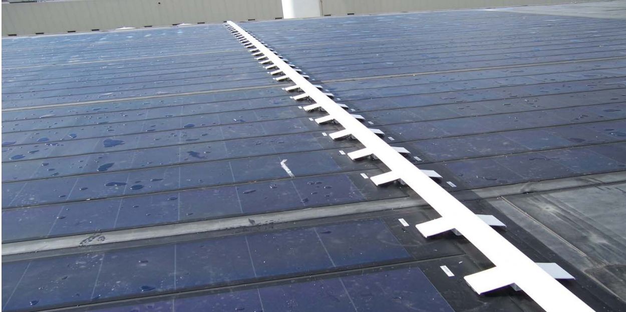
Figure 39: Installed UNI-SOLAR PowerMembrane Array
