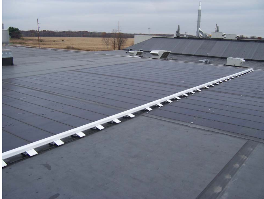
Figure 30: PVC WMS Installation
