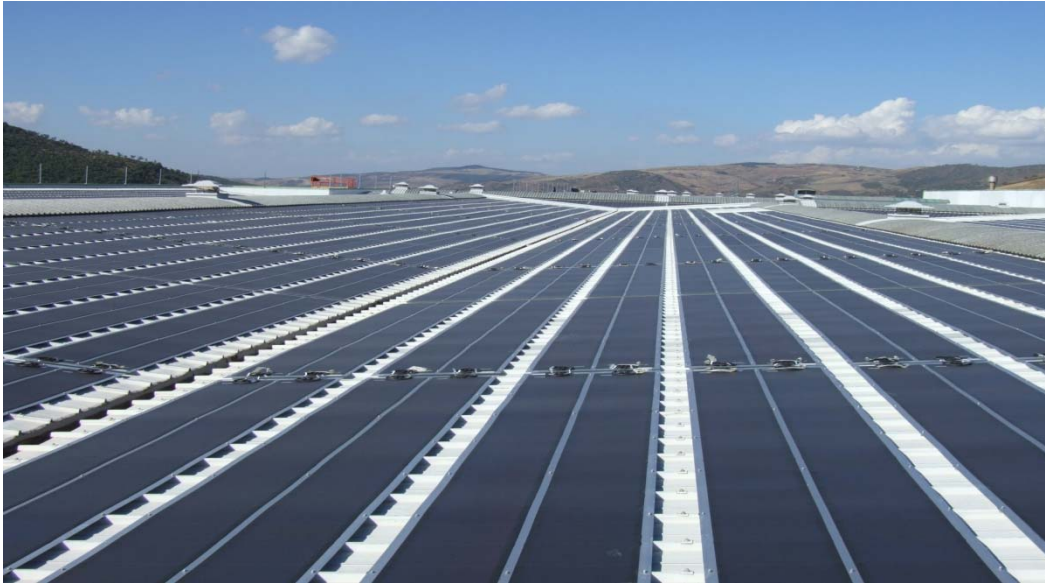
Figure 16: Reference Project Photo for Standing Seam Metal Roofs Not Suitable for Direct Bond
