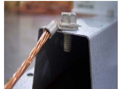
Figure 46 Copper Grounding Wire
