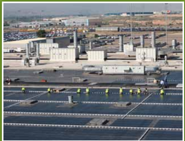
GM Opel Plant | Zaragoza, Spain | 12MW
