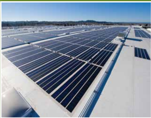
ProLogis | Portland, OR | 1.1MW
