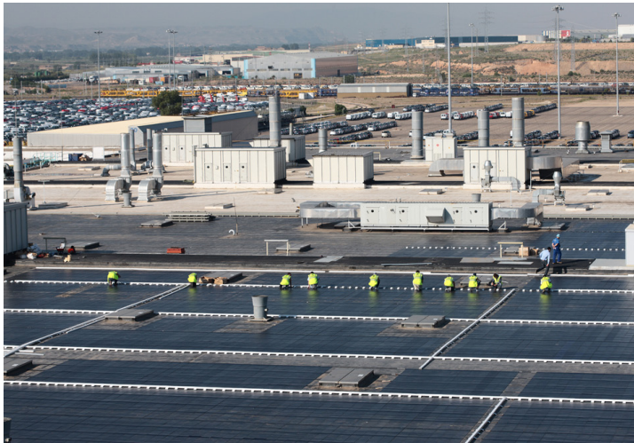
General Motors Facility (11.8 MW) • Zaragoza, Spain World's Largest Rooftop Solar System
