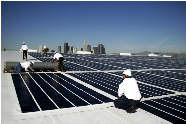
Coca-Cola Plant (329 kW) • Los Angeles, California Installed by, and Photo Courtesy of, Solar Integrated Technologies
