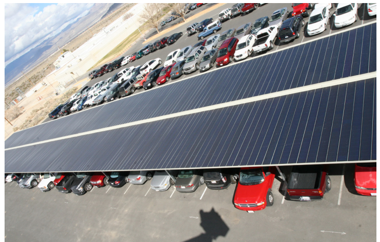
Naval Air Weapons Station - Carport (110kW) China Lake, California
