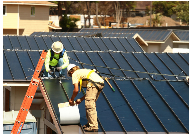
Army Hawaii Family Housing LLC (6 MW) Schofield Barracks, Oahu, Hawaii Actus Lend Lease
